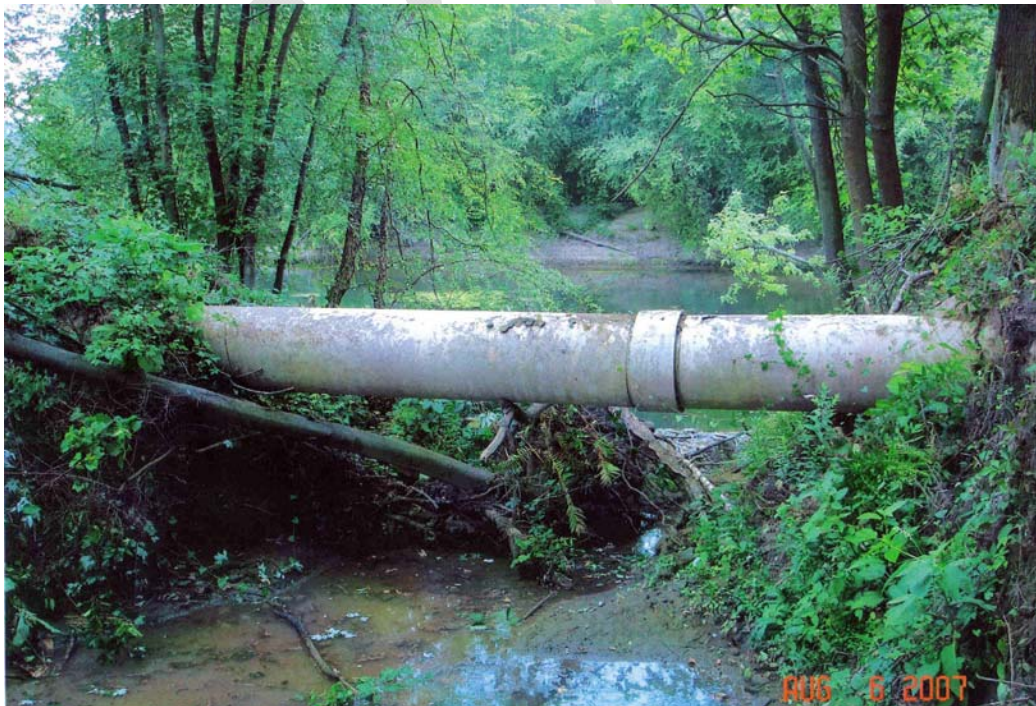
Sewer Washout near Esopus Creek, Town of Ulster
